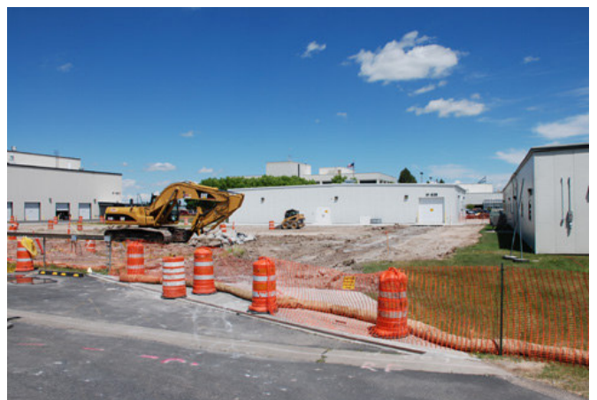
Photo depicts progress on the site of new RESL Annex in Idaho Falls as of early June 2010.
